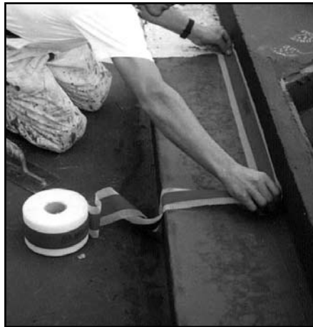
An example of Mapeband waterproofing a corner between the bottom and a side of a bathtub
